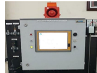
Surveillance and Safety
