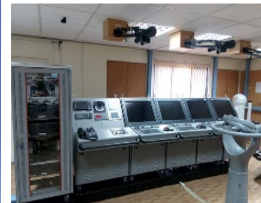
Navigation & Bridge System
